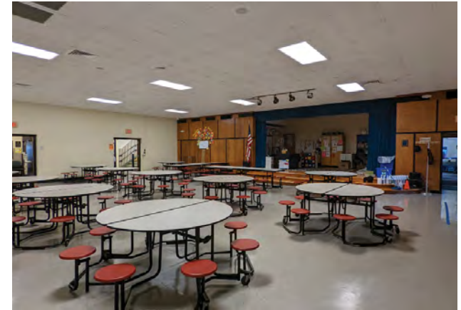
Cafeteria with stage; stage is inaccessible (no ramp, only accessed via stairs)
