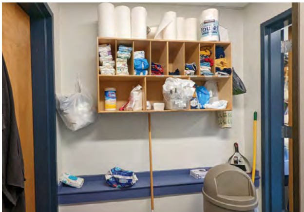
Shared toilet room; inequitable distribution of toilet facilities for classrooms
