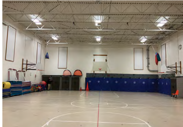
Undersized gymnasium with no spectator seating/bleachers and inadequate storage
